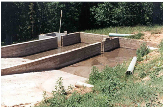
Figure 4–2 Two settling basins arranged in series treating liquid dairy manure with adjustable-height weirs (Clemson University Extension)
