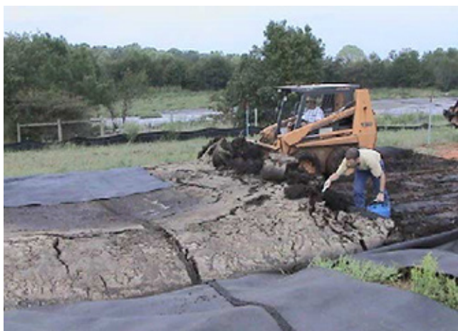
Figure 4-68 Unloading a small geotextile tube used to dewater dairy lagoon sludge (University of Georgia Cooperative Extension Service, Worley et al., 2004)
