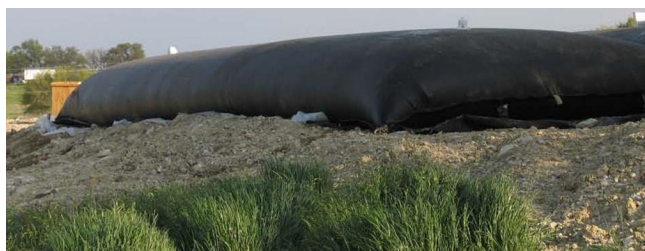
(b) Geotextile tubes used in Texas with alum and PAM enhancement (14 ft wide × 50 ft long).
