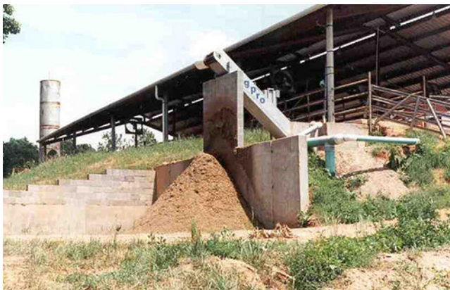
Figure 4–9 A small in-channel flighted conveyor separator installed above the solids stacking area (Clemson University Cooperative Extension)
