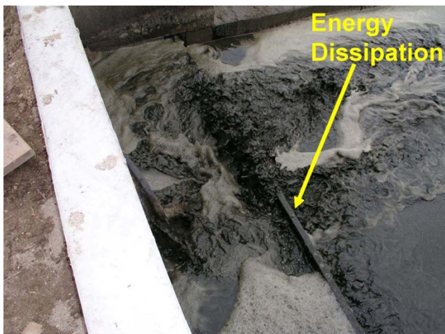
Figure 4-48 Short baffle used to dissipate energy and spread influent to a sand lane (University of Wisconsin, Cooperative Extension Service, Holmes, 2010). Other materials that can be used include poured concrete curb or concrete block attached to slab by filling cores with concrete around steel bars set in the slab
