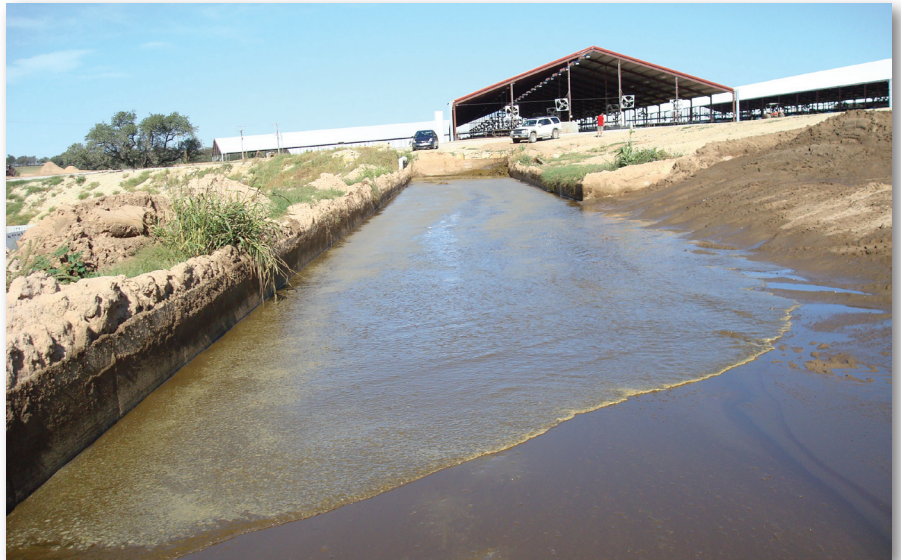
Final effluent leaving the chambers of the secondary weeping wall. This liquid is conveyed to lagoons for storage and treatment. Lagoon liquid is then used for flushing the manure alleys in free-stalls.
