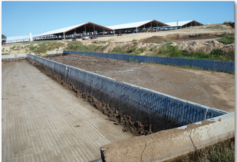
Looking upstream at the primary weeping wall. The sand settling lane runs along this weeping wall. The ramp to remove settled sand from the channel, and the recovered sand (foreground) and the stockpiled dried sand to be recycled as free-stall bedding are visible in this picture.
